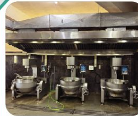
Fresh Air Ducting
