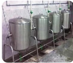
Steam Cooking Line Tata c Pipe
