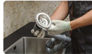
Break down maintenance
