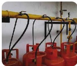
Commercial Kitchen Gas Pipeline
