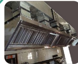
Hood with Filter and GI Ducting
