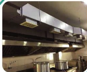
Fresh Air Ducting
